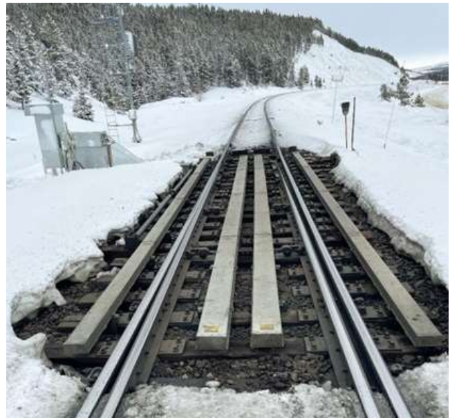
Figure 4. Installed Hellfire clears snow and ice. Source: Thermon, Inc.
